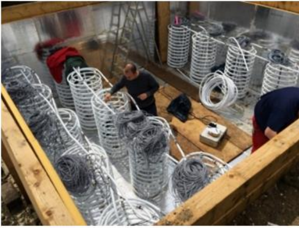
Fig 1 Installation of helical heat exchangers and temperature sensors in the excavation pit for the storage.
