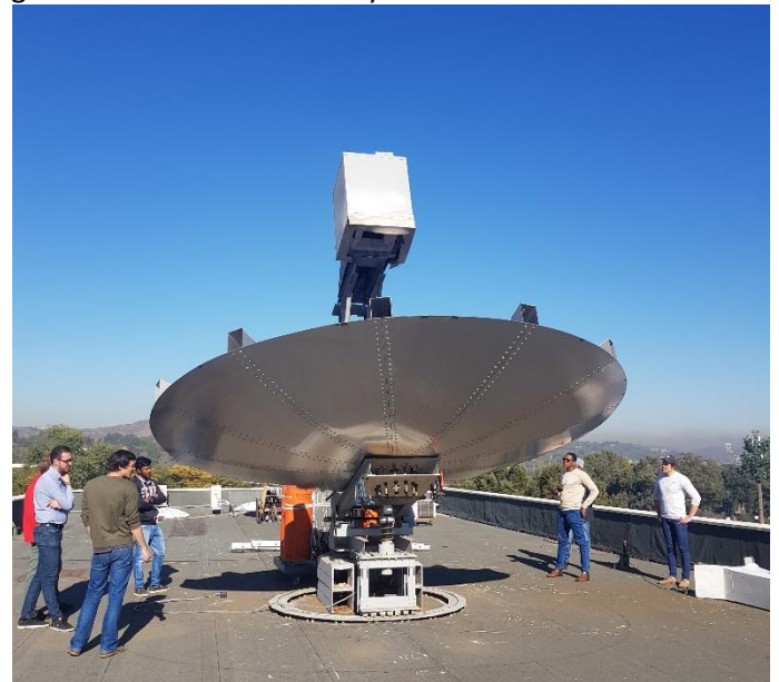
Fig 1: SSBC installation at the University of Pretoria.
