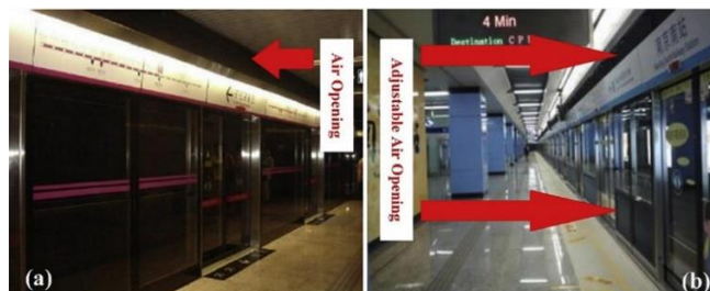
Fig. 4. (a) Platform Bailout Doors system (PBDs). (b) Adjustable Ventilation Platform Doors system (AVPDs) [20].
