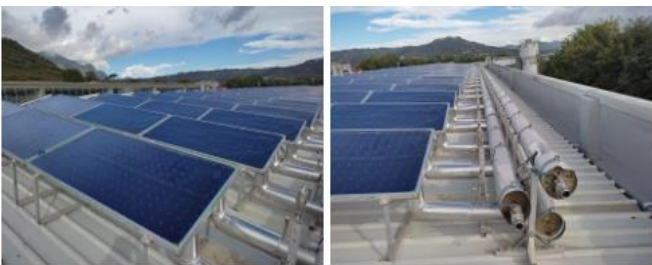
Figure 3 Solar Field test-facility on the roof of TVP-Solar company
