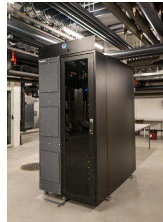
Fig. 3. Picture of the small-scale (12 kW) edge data center installed in NEST within the framework of Eco-Qube project [4]
