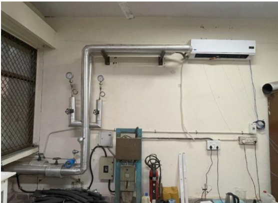
Fig. 3 Installed TES-FCU system at the heat transfer lab, IIT Delhi.
