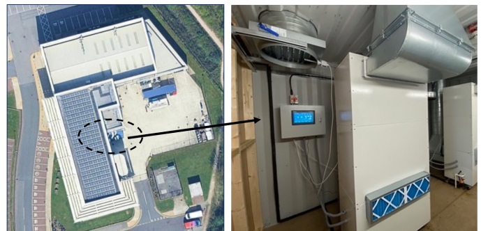
Figure 2 The DPC units at AIC in Hessle HU13 OGD
